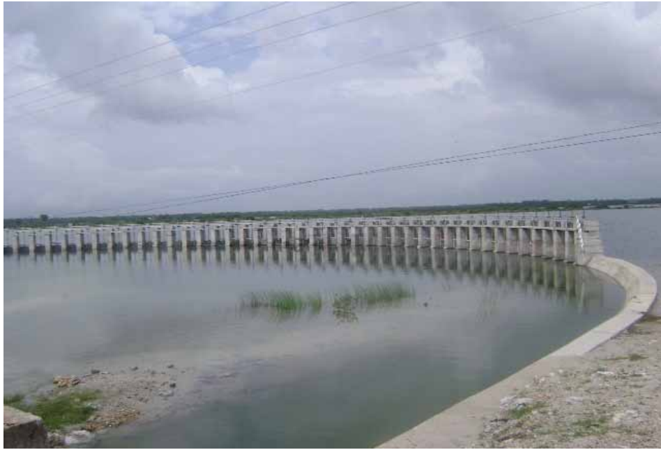
Figure 40. Barrage across Uppu Aru Lagoon at Navanth Kuli Bridge in the Jaffna District.
